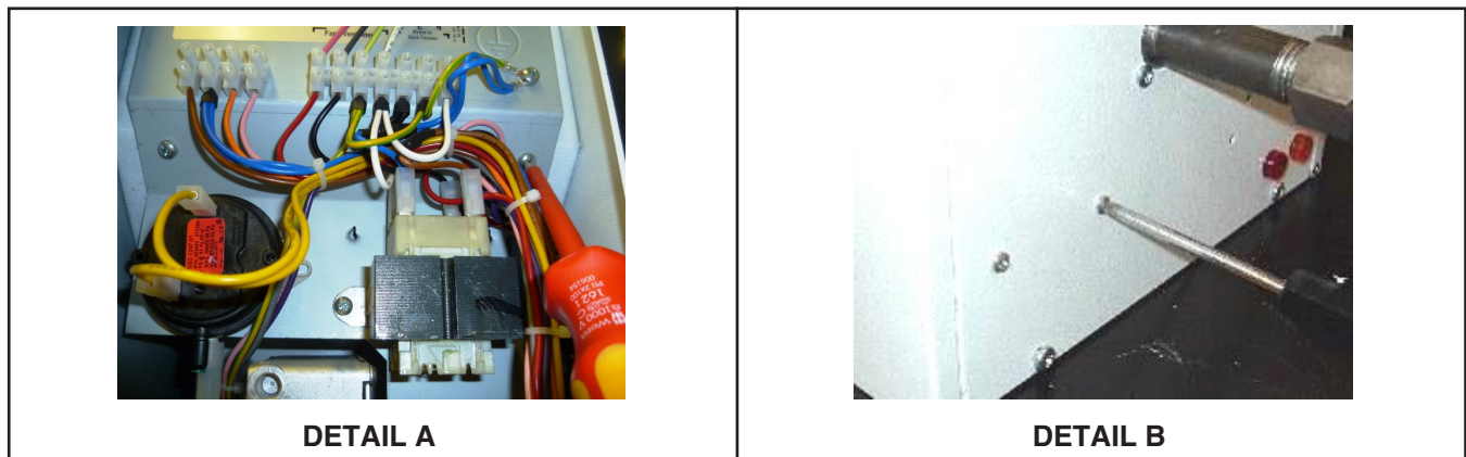
Figure 29. Pressure Switch Removal
